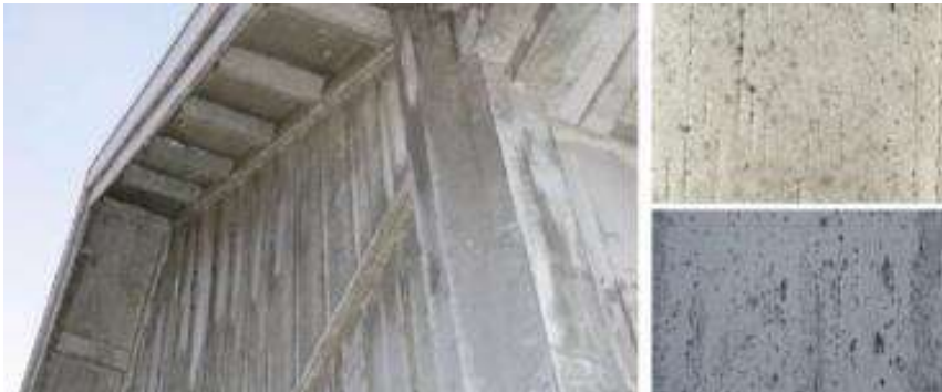
IMAGEN 8 Wooden façade with the signs of moulds growth. Images courtesy of Lone Ross Gobakken, NIBIO
