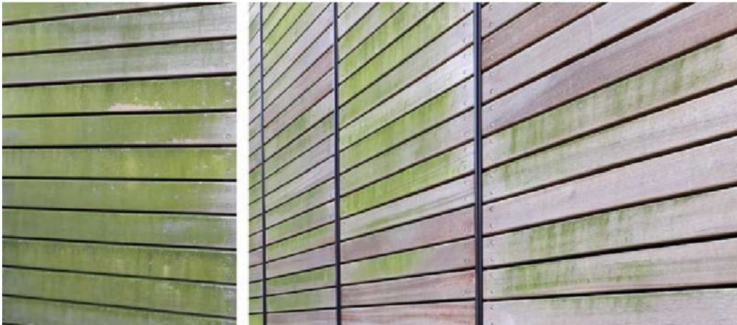
IMAGEN 9 Algae growth on the building façade P
