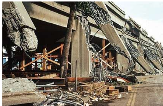
Figura 1.6 Freeway Cypress, Oakland, CA.
