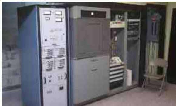
Ilustración 46: Transmisor Nautel: http://www.engineeringradio.us/blog/wp-content/uploads/2011/02/Nautel-ND-5-transmitter.jpg
