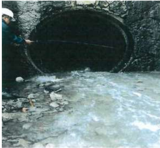
Figure 1.3: Undermining Paso Expres Culvert
