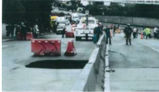
Figure 1.2: Undermining Paso Expres
